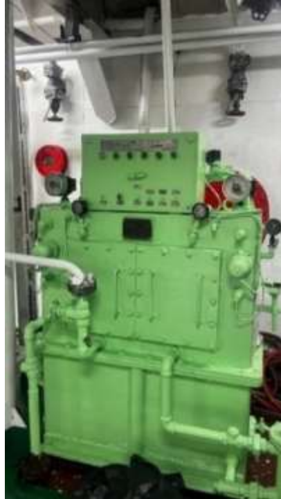
Gambar 2. 2 Oil Water Separator (Sumber : Penulis, 2025)
