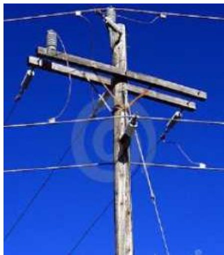
Gambar 2.8 Wooden Pole Tower
