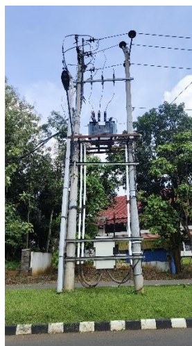
Gambar 2. 1 Gardu Distribusi Tipe Portal
