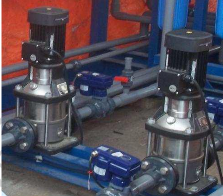
Gambar 2.22 BWRO Feed Pump with Vertical Driven Motor
