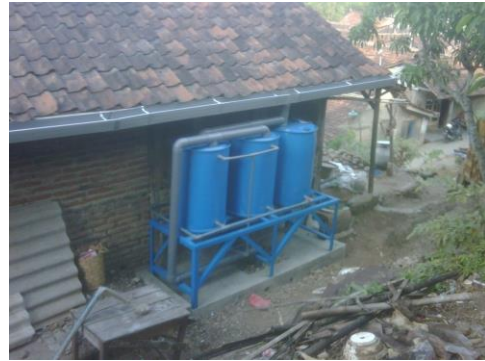
Figure 2. Installed RH Facility in Household.
