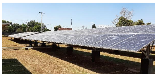
Gambar 2. Gambaran Modul Surya PLTS on Grid 50 kWp UPDL Makassar
