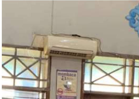
Gambar 4.6 Air Conditioner Perpustakaan
