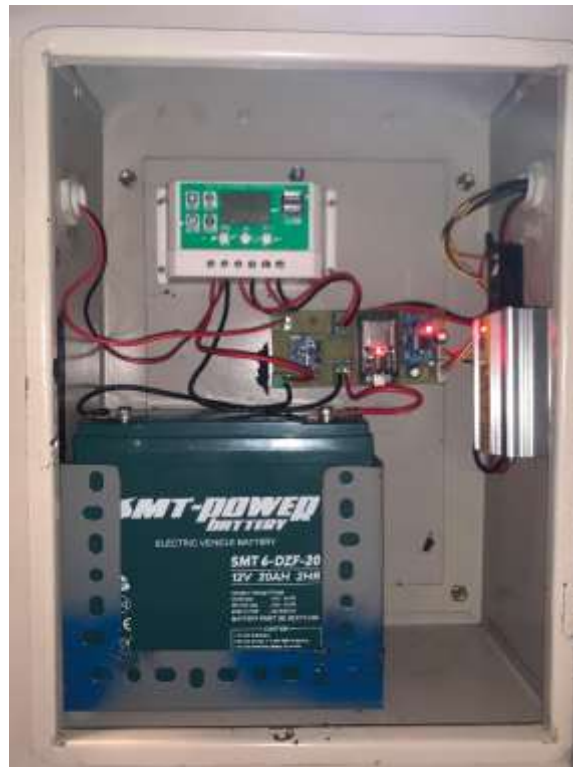
Gambar 4. 4 Integrasi Sistem Monitoring Panel Surya
