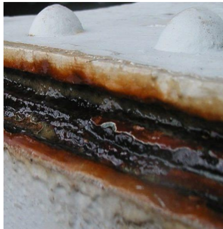
Gambar 2. 7 Crevice Corrosion (Sumber: orapiasia.com , diakses 2026)
