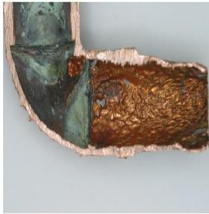
Gambar 2. 3 Errosion Corrosion (Sumber: Utomo, 2009)
