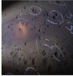
Gambar 2. 2 Pitting Corrosion (Sumber: Microbiology, 2011)
