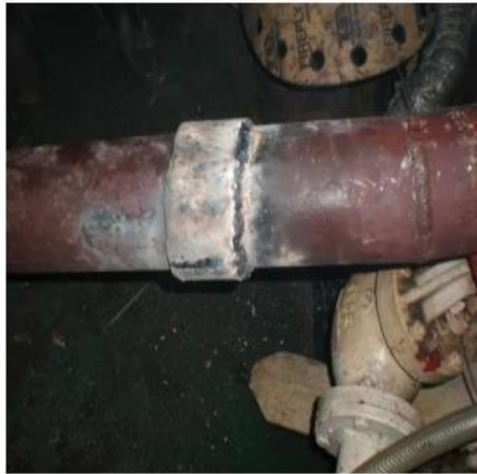
Gambar 2. 4 Galvanic Corrosion (Sumber: Utomo, 2009)
