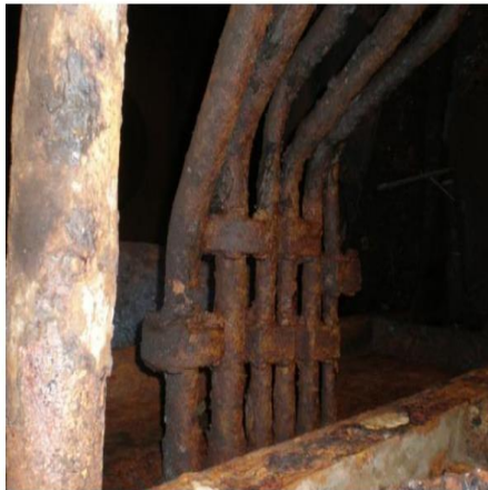
Gambar 2. 5 Unifrom Corrosion (Sumber: Utomo, 2009)
