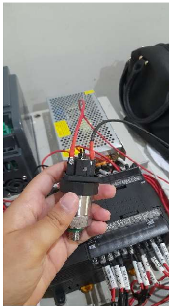
Gambar 4.3 Pengujian Pressure Transmitter
