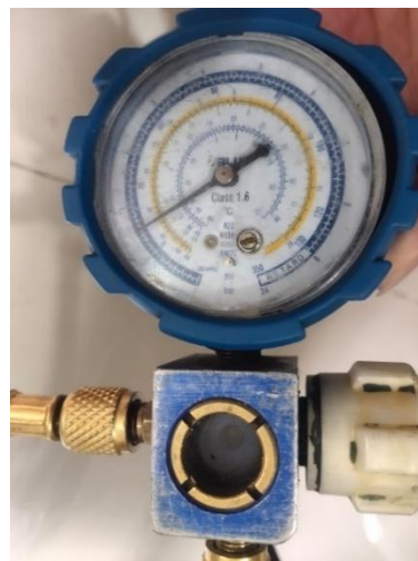
Gambar 4.18 Hasil Pengukuran Manifold Gauge
