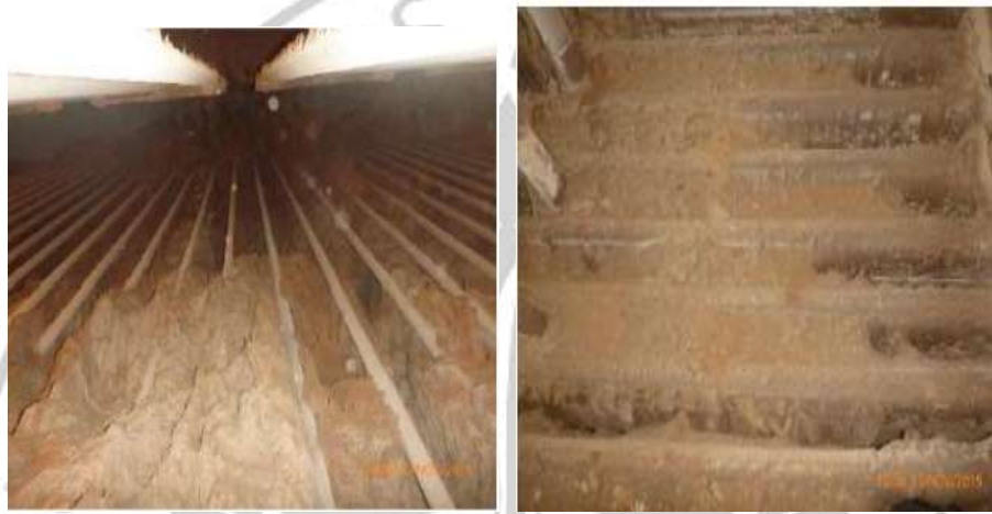
Gambar 2. 7 Fouling di area boiler backpass (MHI, 2022)
