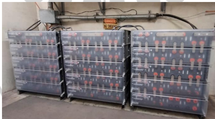
Gambar 2.6. Baterai Emergency Sumber: PLTU XYZ
