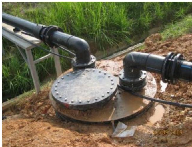
Gambar 2.29 Tank Drainase Air Lindi
